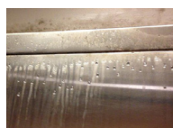
Figure 2. Visible condensation on cold room door.
