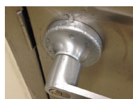
Figure 3. Visible condensation on cold room door handle.
