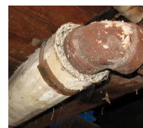
Pipe Insulation - Friable
